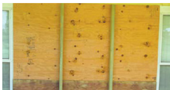
Figure 4-20. Plywood cut to protect sliding glass doors, supported with two 2x4s and attached with screws. (Source: Hawaii Sea Grant)
