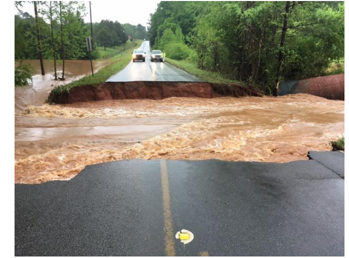
Figure 2-13. A road that was washed out from flash flooding in Troup County, Georgia. (Source: National Weather Service)
