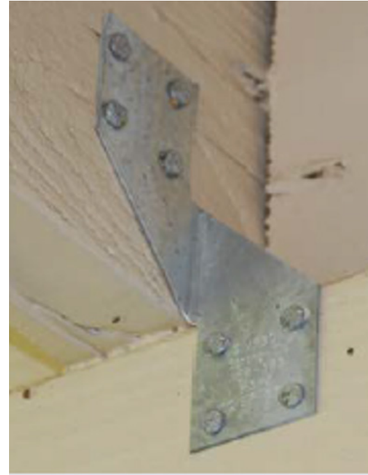
Figure 4-25. Hurricane clip on a retrofit. (Source: Hawaii Sea Grant)
