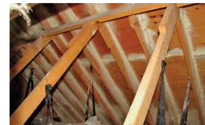
Figure 4-5. Spray foamed attic, used to strengthen rafters and plywood sheathing supporting the roof. (Source: FEMA)
