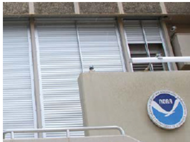
Figure 4-18. Rolldown shutters protecting windows at a NOAA National Weather Service facility. Two shutters are fully deployed and the remaining are partially deployed. (Source: Hawaii Sea Grant)
