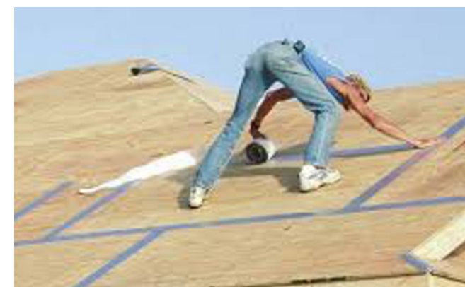
Figure 4-4. Water intrusion tape being applied to roofing seams to prevent leaking. (Source: FEMA's "Local Officials Guide for Coastal Construction")
