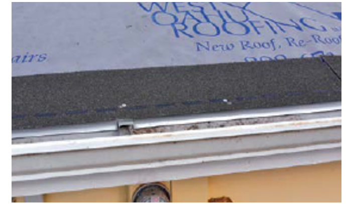
Figure 4-8. Roofing felt tacked on to the self-adhering modified bitumen layer. (Source: Hawaii Sea Grant)
