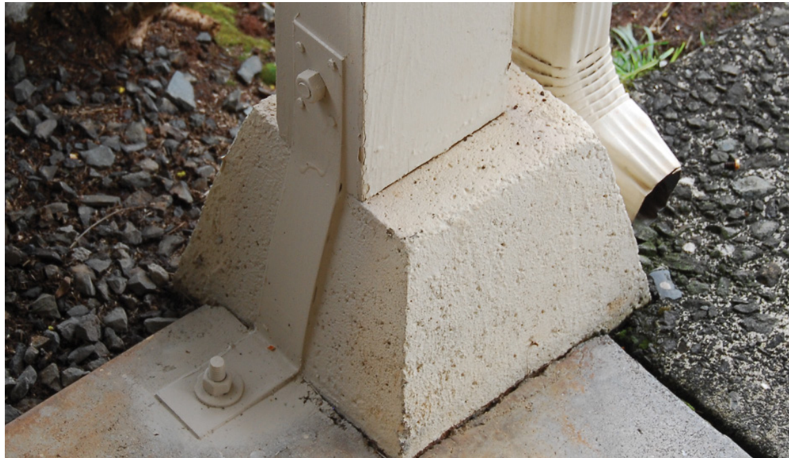
Figure 4-1. Example of retrofitting by connecting a piece of the house to the foundation. This is an example of attempting a continuous load path connection from the roof to the foundation. (Source: Hurricane Protection Services)
