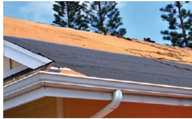
Figure 4-7. A self-adhering, modified bitumen layer acts as a synthetic underlayment material on top of the initial plywood layer. (Source: Hawaii Sea Grant)
